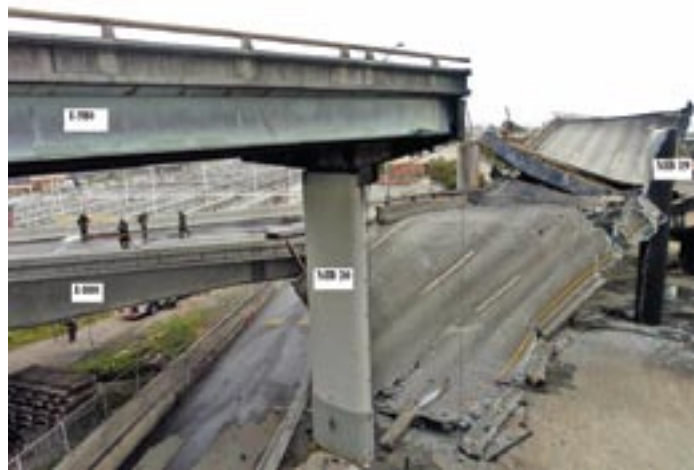
Two spans of I-580 collapsed onto the I-880 connector ramp directly below.
