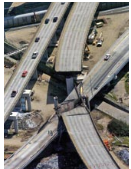
The steel box beam bent cap spanning the I-880 connector collapsed in the estimated 1,500 °F fire.
