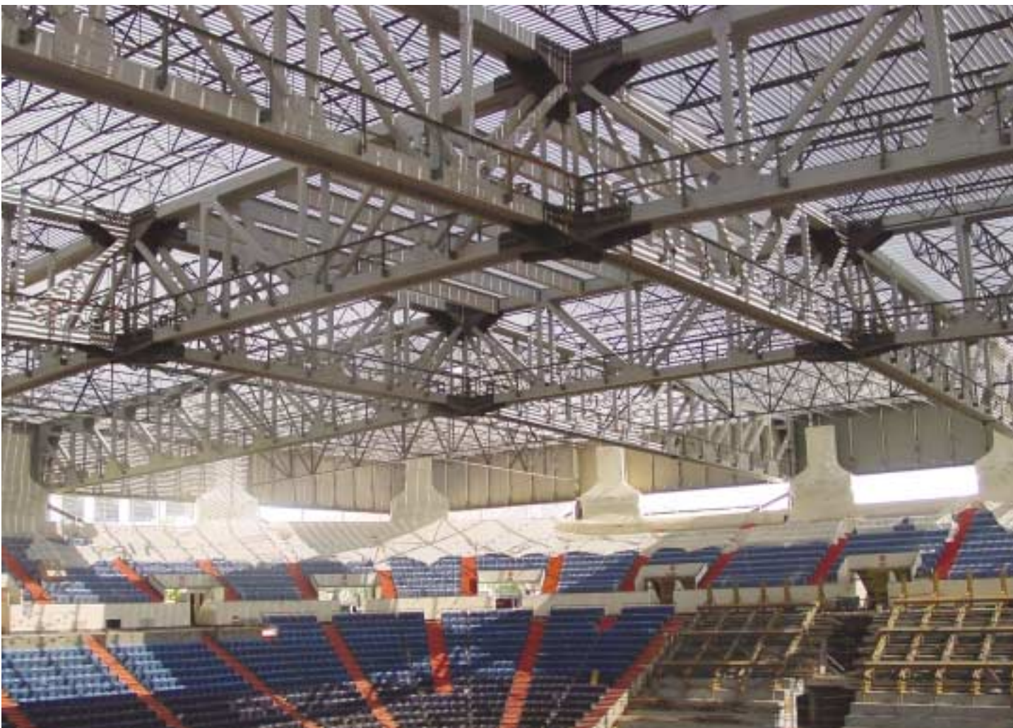
Below: View from inside the arena looking up after the roof deck was installed. Note the "built-in" catwalk system. The joists are oriented in perpendicular directions in adjacent bays.
