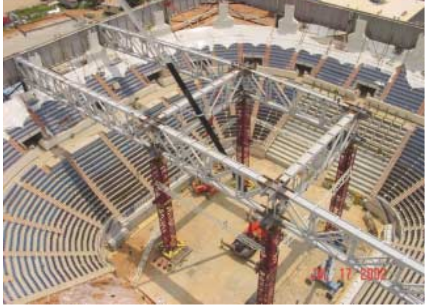
Overhead view of the main trusses during the erection stage. The four shoring towers were used both during demolition and erection.
