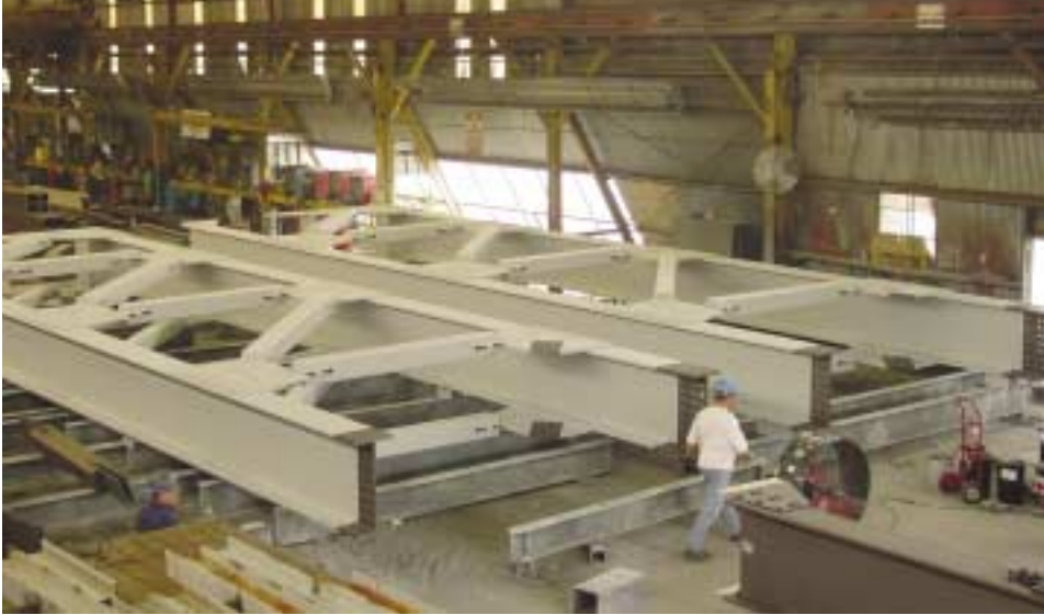
Opposite page: An aerial view of the last of the 120' truss sections being put in place.
